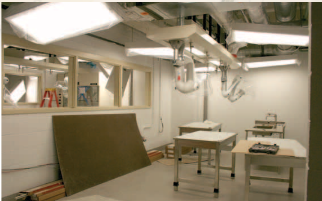
Construction of one of three nearly identical manufacturing laboratories where students and faculty will be able to view one another through a wall of windows that separates these spaces
